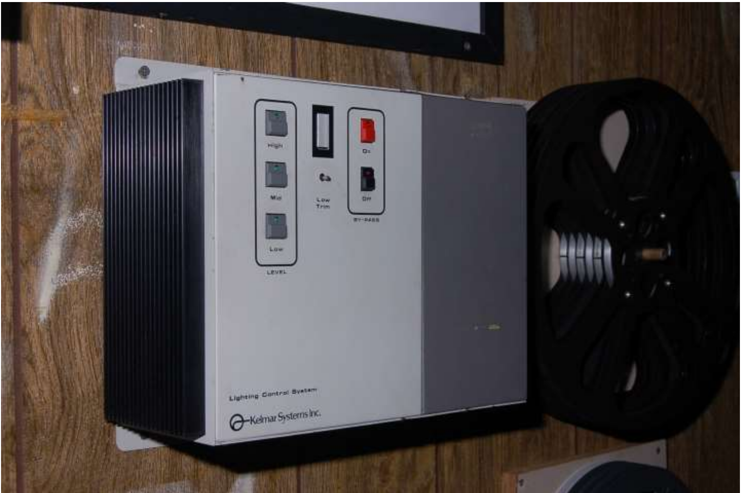
A Kelmar theater dimmer. One from a multiplex! Soon to be connected and fading away! You don't get these at the big box stores!
